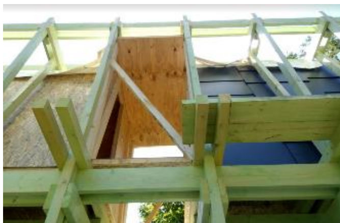
Fig. 26 During the installation of upper floor, the stretching double beams provided space for scaffolding.
