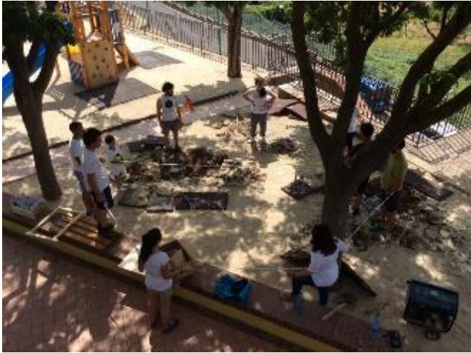
Fig. 11 The group works with the tutors and the carpenter to dimension the structure and to place the tree passing from inside the playground.
