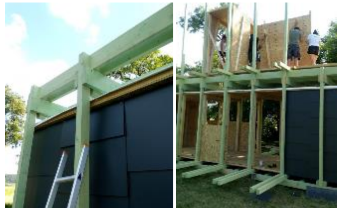
Fig. 25 The cladding of the side façade and the installation of upper floor wall panels.
