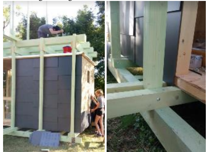
Fig. 24 The cladding of the façade and the detail of joints at the base.
