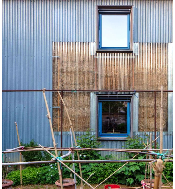
Fig. 15 Sarah Wigglesworth and Jeremy Till, Strawbale House , Islington, North London (finished in 2001). Wing with walls having wooden structure, straw bale infill, corrugated sheet metal and polycarbonate cladding.
